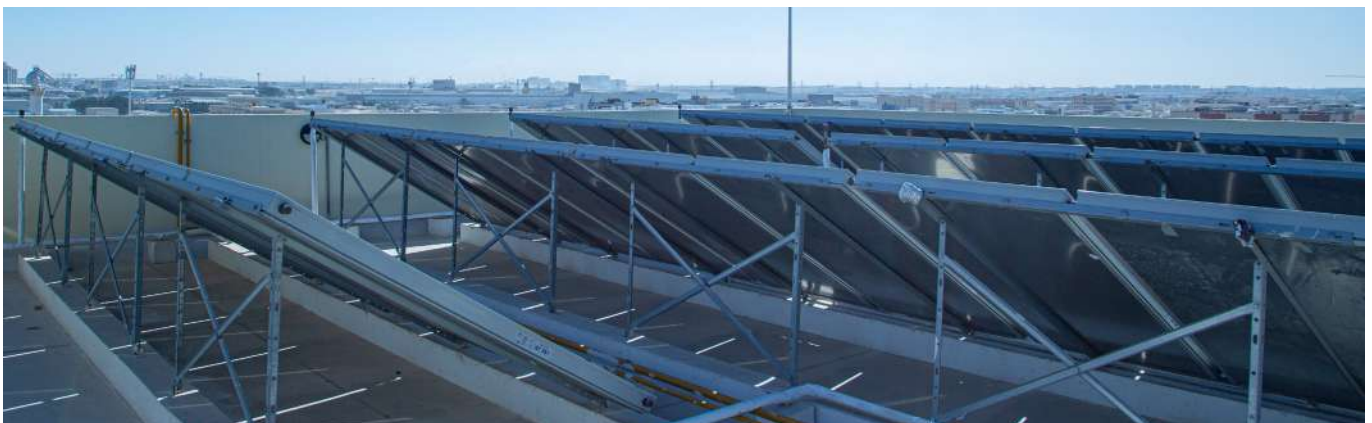
Solar panels at the top of one of our accommodations in Jebel Ali.
